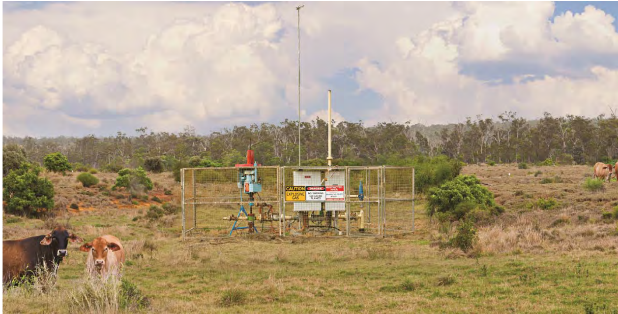
Plate 20-27 Production Well Head (Source Arrow)
