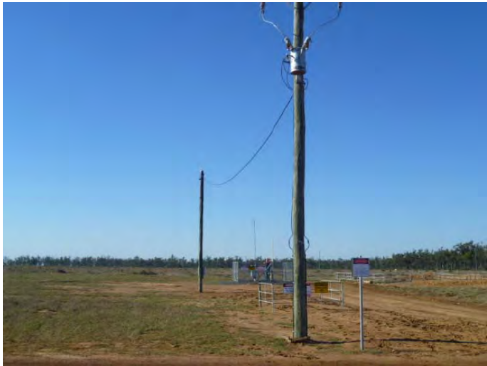
Plate 20-26 Overhead Power Line to Well Head (Source Arrow)
