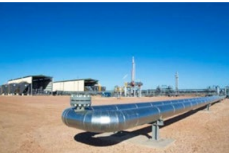
Plate 2. Central Gas Processing Facility
