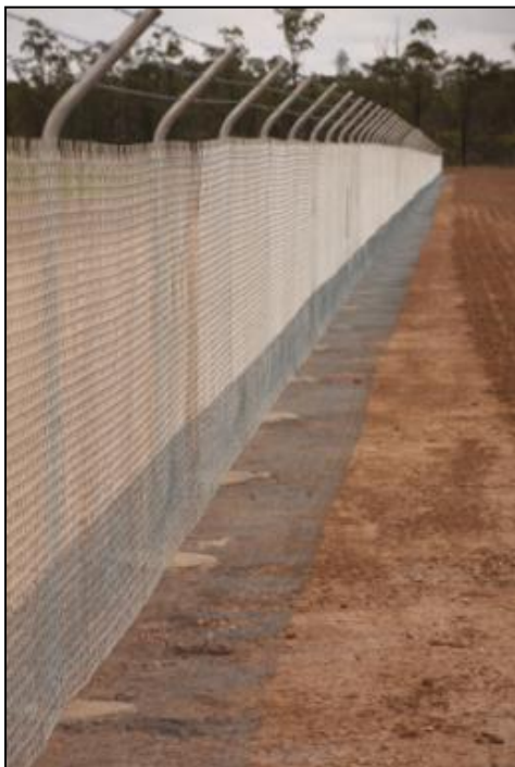
(Left) Floppy bottom fence at Punchbowl Pilot Dam with barbed wire top
