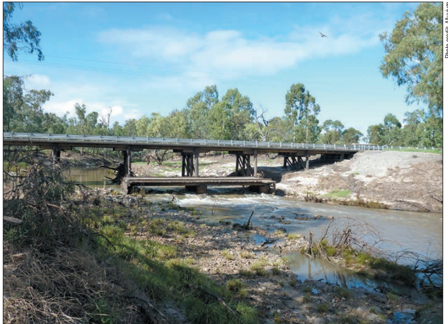
Plate 9.11 The Toowoomba Cecil Plains Road bridge in reach 6 of the Condamine River
