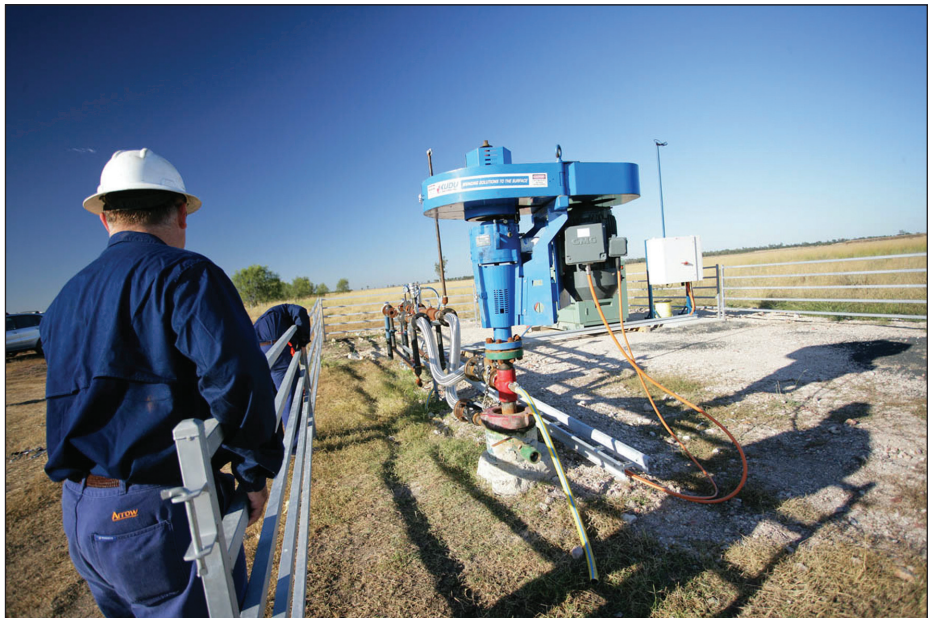
Plate 5.5 Well site pump
