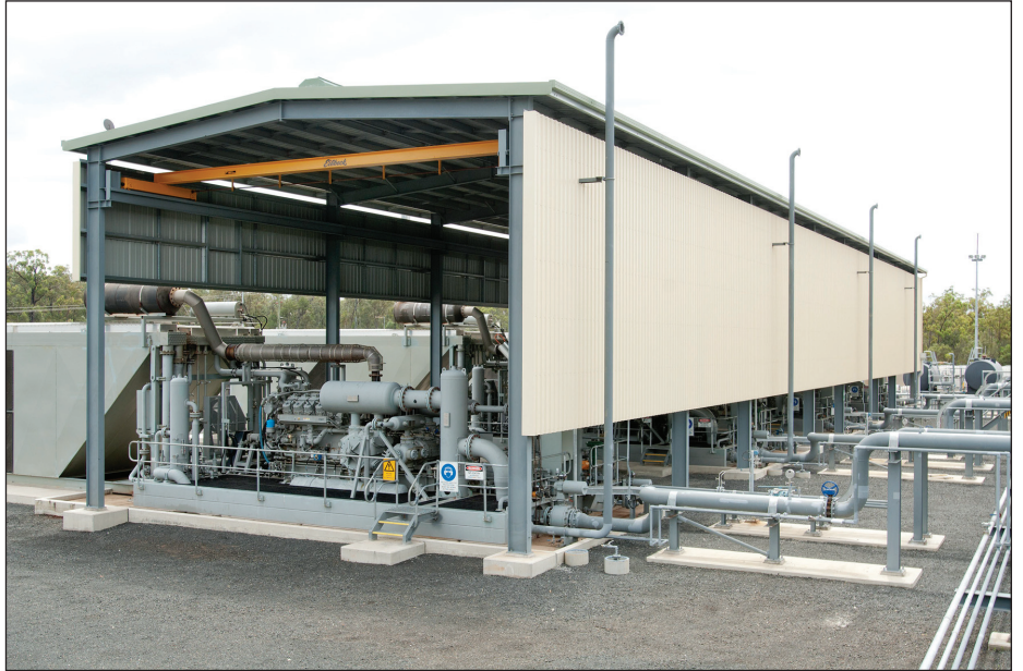
Plate 5.1 Gas compression facility
