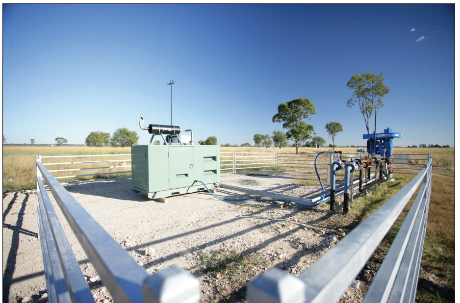
Plate 5.3 Well site generator
