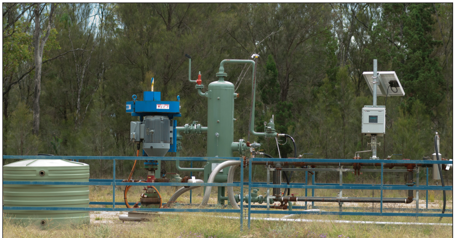
Plate 5.8 Production well surface facilities
