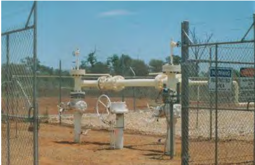
Plate 3-46: Typical enclosure around a valve on a rural property
