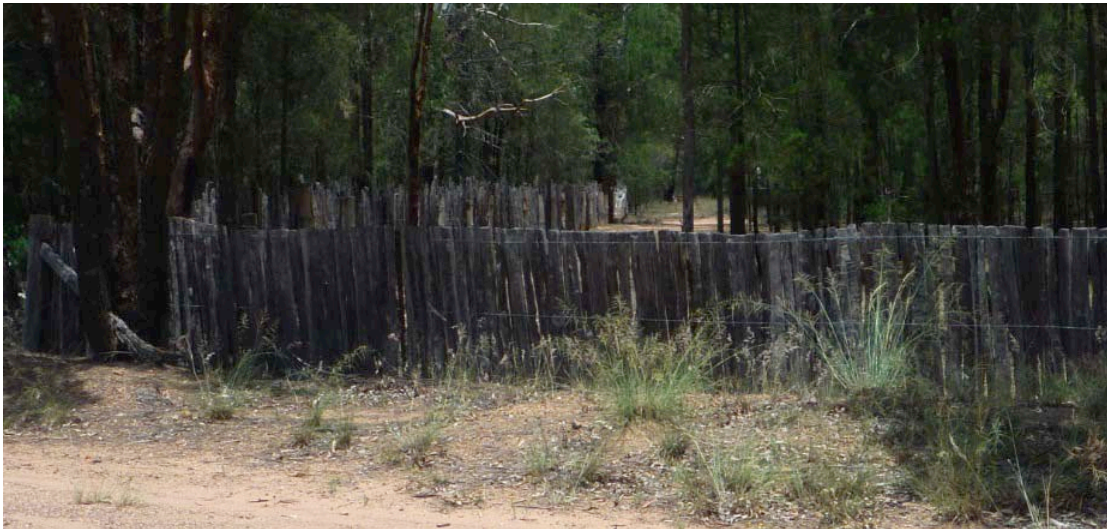
Close-up of fence 2 shows original section around the corner. The section at the front has been rebuilt and reinforced with barbed wire.
