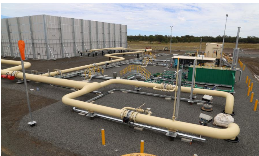
Harry Inlet Processing facility – newly constructed 27km SW of Dalby. Approximately 180 Arrow staff, contractors and sub-contractors worked on the project
